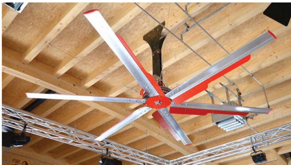
Figure 7. Ceiling fan for the control of the temperature in barns. The fan is fitted with five or six aluminum blades. The diameter of the fan varies from 3 to 5 m depending on the size of the barn.
